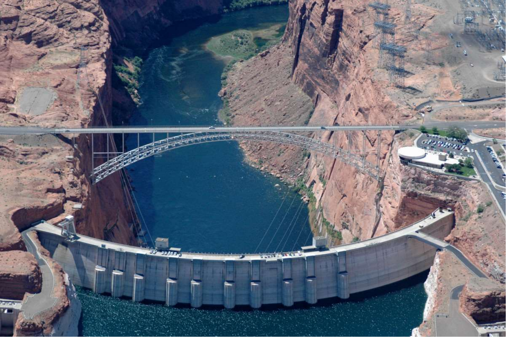
Top: Glen Canyon Dam is located on the Colorado River in northern Arizona, near the town of Page. (Photo: Arizona OpsEval Mission Aircrew)
